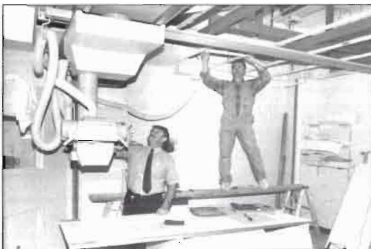
Chief Radiographer, Ian Channing and Building Contractor, Peter Skyrpko, working on the installation of the new radiology equipment.
