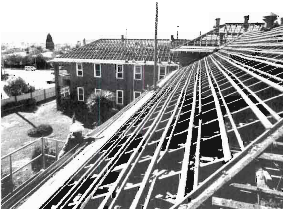
Demolition of the Hutton-Jones and McDonald Wings of the nurses home begins in preparation for the commencement of the Redevelopment Program.
