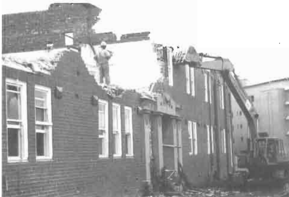
The redevelopment begins with demolition as workmen tear down the Hutton-Jones and McDonald Wings of the old nurses home.
