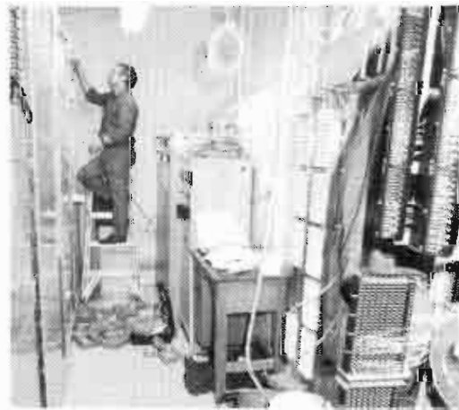
Installation of the new SPC PABX.
