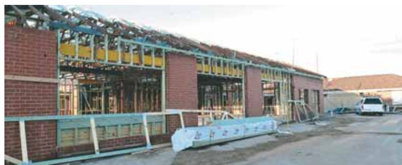
Above: Building works commence on the new Community Rehabilitation and Oncology Centre.
