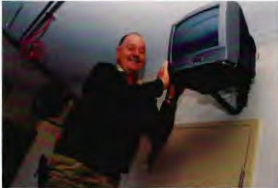
Paul Tangey from the Maintenance Department installing new television sets during the redevelopment process
