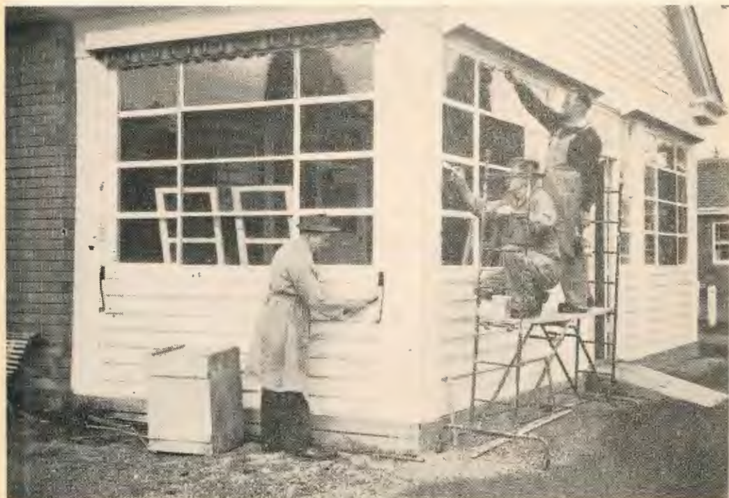
Maintenance Staff Messrs Stan Hair, Jim Seary and Ted Maddocks carrying out repairs to one of the balconies
