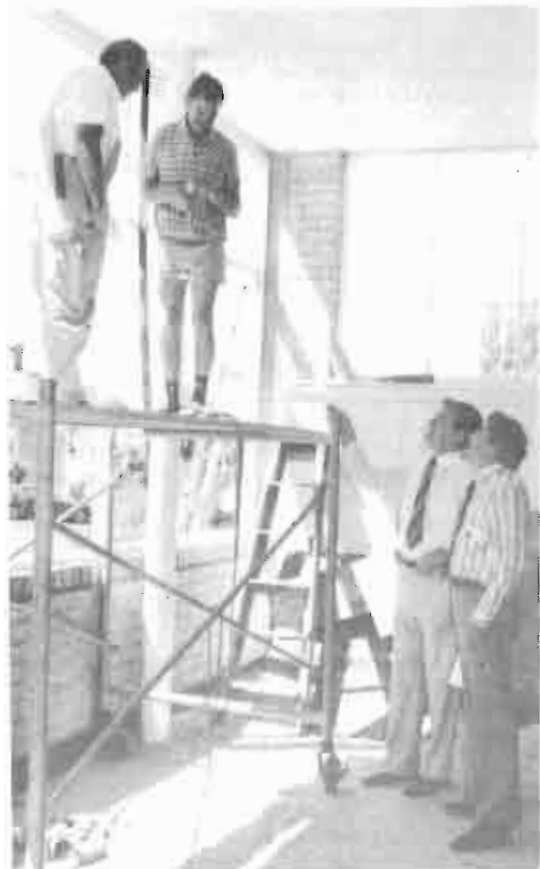
The Chief Executive Officer, Mr. E.D. Macaulay, and Mr. Tom Evans, MLA inspect the progress of the renovations in the Urology Unit. The full cost of the work was met by the State Government under the Minor Works Programme.
