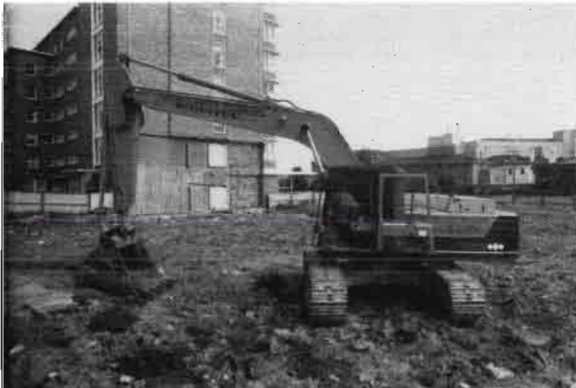
After demolition of the Old, the machinery moves in to commence the New.
