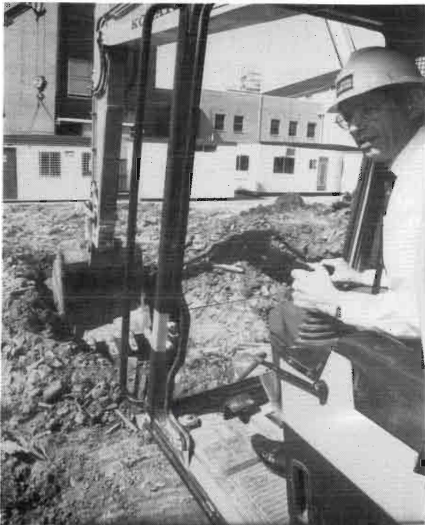
Mr. Derek Woolley, President of the Board of Management officially turns the first rod for Phase One of the Hospital's Redevelopment Program.
