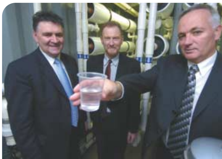
Central Highlands Water managing director, Neil Brennan, Eureka Linen's manager Paul Robinson and Ballarat Health Services CEO Andrew Rowe with some recycled water.
